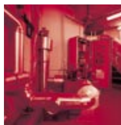
■ Air conditioning units
